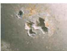
Surface damage inside a ship's diesel oil tank
